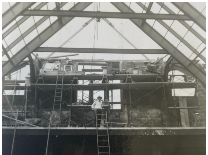
1959-60 construction of the long-awaited new church, located west of the school and rectory
